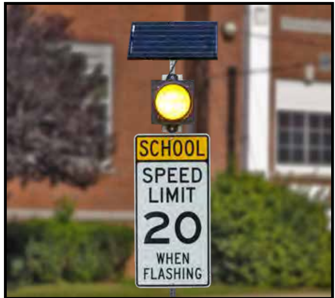
School Zone Flashing Beacon
