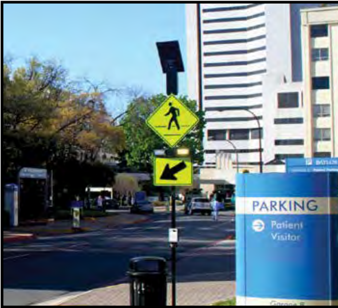
Solar Powered Rectangular Rapid Flashing Beacon
